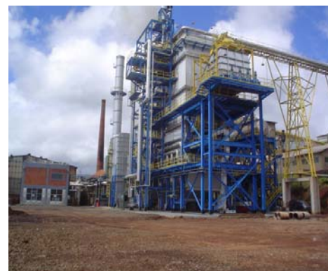
The biomass facility at Irani.
